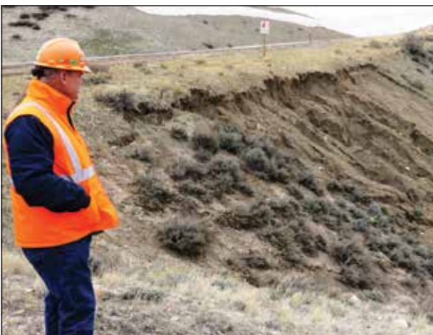
Wyoming Department of Transportation District Engineer Pete Hallsten of Basin views one of the moisture slides at milepost 45.5 on Chief Joseph Highway near Cody.
